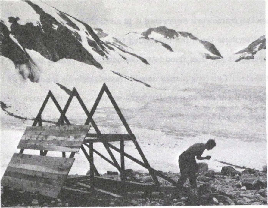
From erection of the A-frame house at Woolsey Glacier 1965 Only three rafters were used for this hut and the picture shows the situation when the roof is being attached. Note that the roof will be extending one foot outside the end walls on either side.
